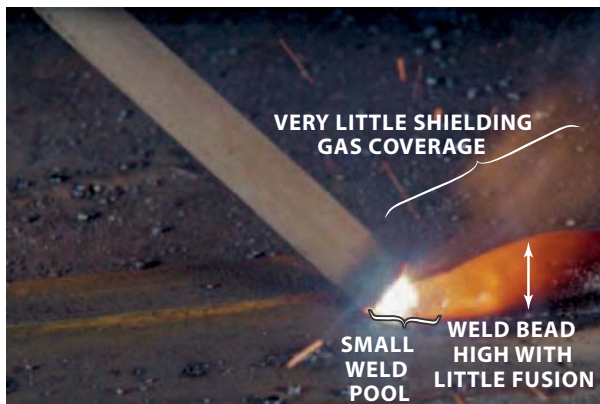
FIGURE 9-2 Welding with the amperage set too low. Larry Jeffus
