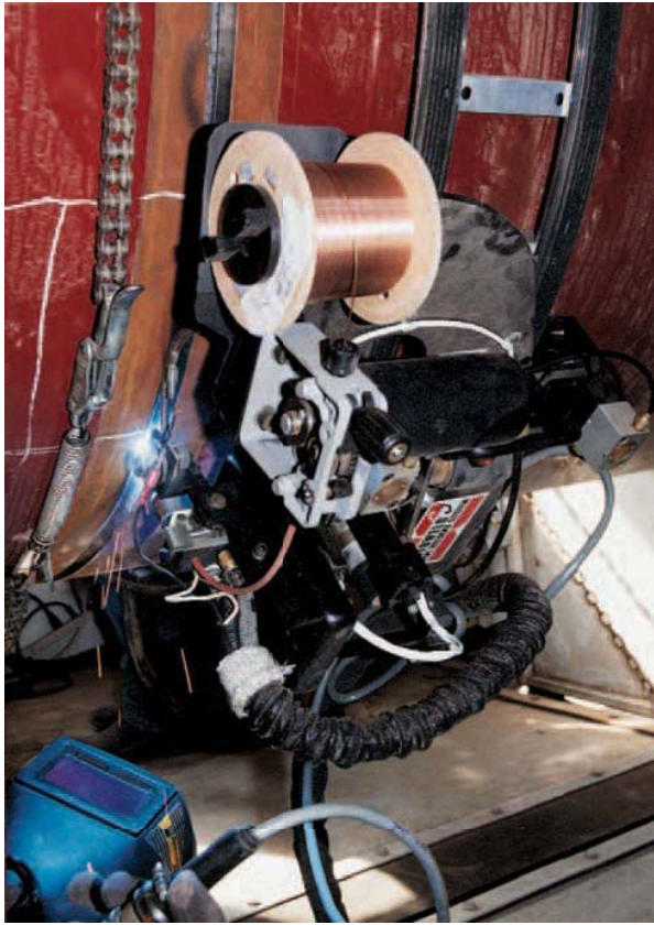
FIGURE 25-9 Automatic GTA machine welding along the seam of a stationary pipe. The Lincoln Electric Company
