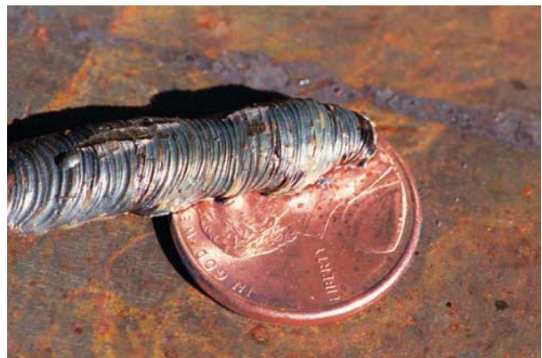
FIGURE 11-31 Weld separated from the plate; there is no fusion between the weld and plate.
